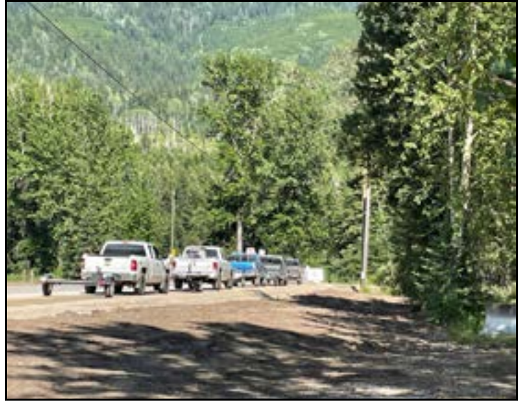
2 - Morrissey Boat Launch parking improvements. Big thanks to RDEK, MOTI and TC Energy to address the safety and parking issue.
